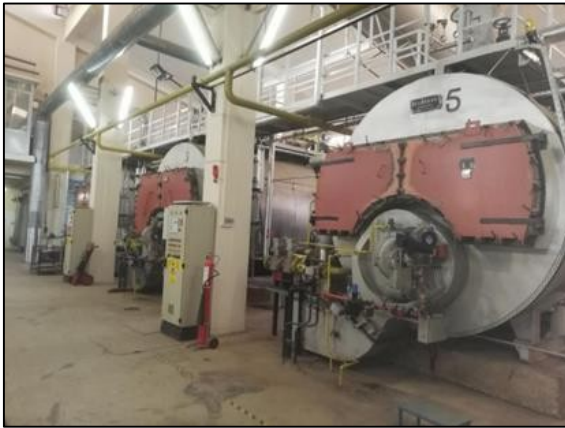
Figure 3. Existing Heating System.
