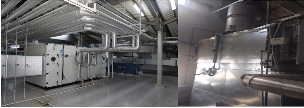
Energy Saving Systems
