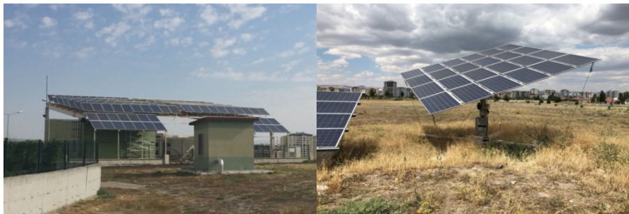
Solar Energy Generating Panels
