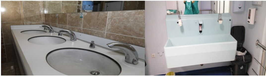
Saving Taps Used in Buildings
